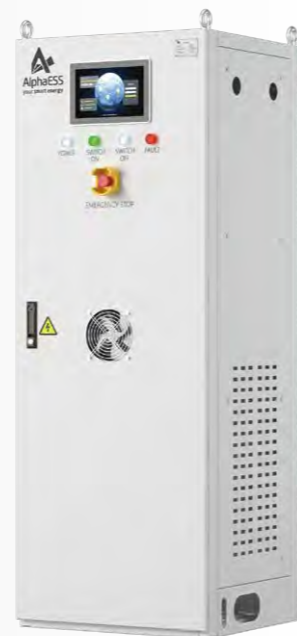
DC Junction Cabinet
